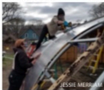
Volunteers Bozena Scheidel and Mattie Wong secure polycarbonate glazing. Volunteers have been essential to the project.
